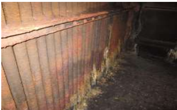
圖 3 2015 年熱交換器管腐蝕狀況 [1] 。 Figure 3 Corrosion condition of the heat exchanger tubes in 2015 [1] .
