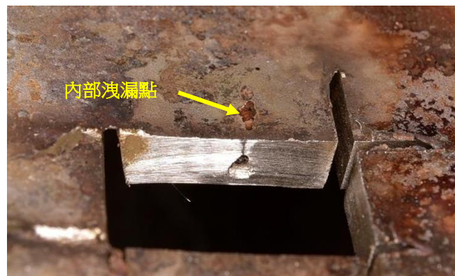
圖 5 洩漏點經截面切割後之外觀。 Figure 5 Cross-sectional view of leak point on the pipe.
