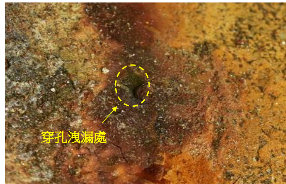
圖 4 圖 3 黃色框選處之近拍外觀，洩漏處被厚實的腐蝕生成物覆蓋。 Figure 4 Magnified-view of yellow zone of figure 3, leak point is covered by corrosion products.
