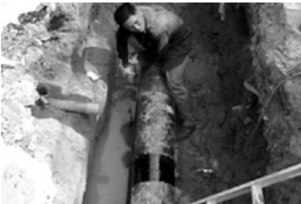
圖2. 破損位置為 12 點鐘方向 Fig.2 Defective position is 12 o'clock direction
