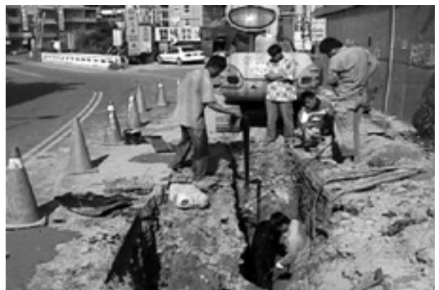
圖6. 管線電位異常 (水泥包覆) Fig.6 Abnormal potential of pipeline (pipelines cased by concrete)
